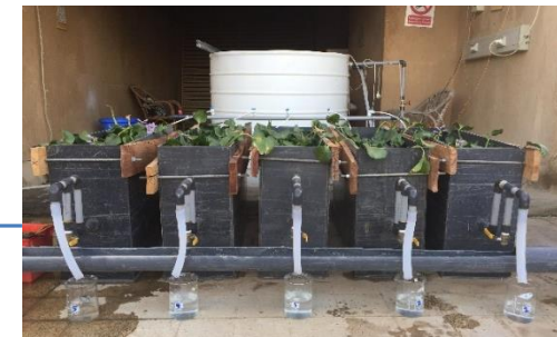
Figure 8- 1: Flow control valves and sampling points
